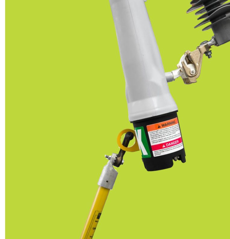
Close Manually Using a Hookstick
